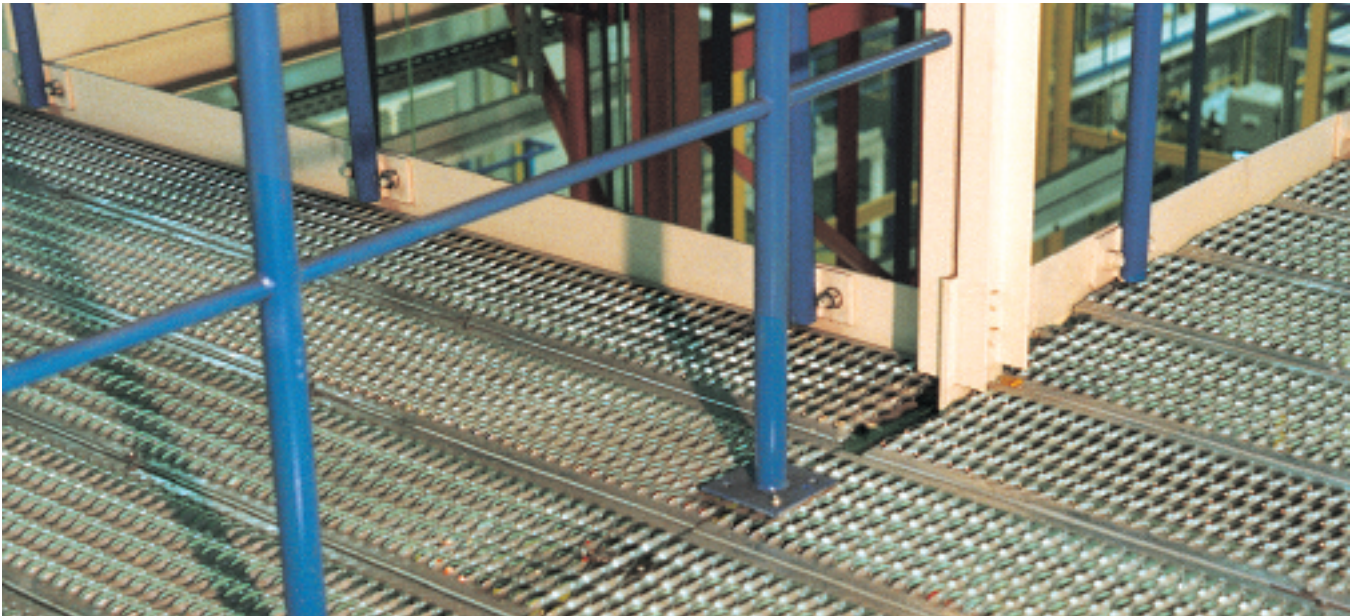
Floor of an intermediate storage hall
